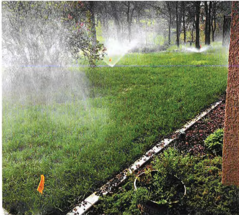
Figure 2.0 Misting caused by high water pressure
